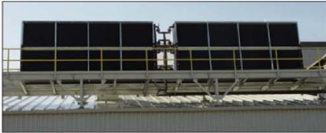
A Large Dry Cooler System
